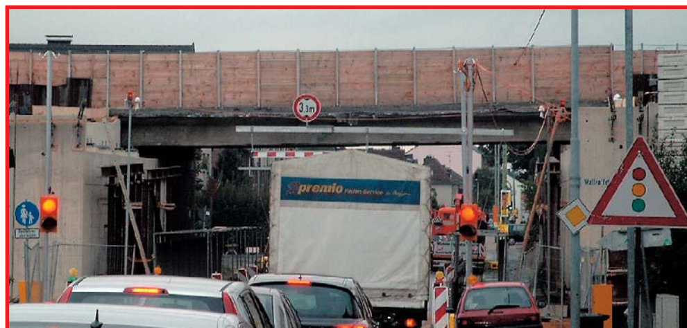
Use of our height warning system at construction work on a bridge in Cologne
