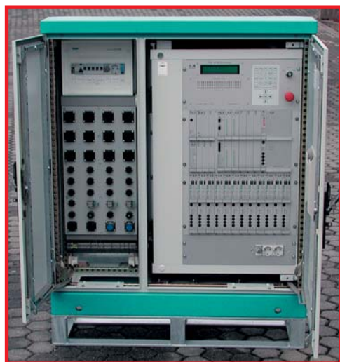
Crossroads control unit EPB 48 Master
