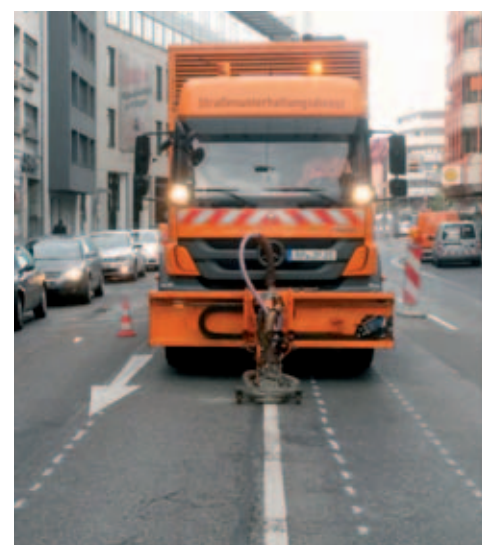
Removing the superfluous marking carefully but thoroughly, without damaging the road surface.
