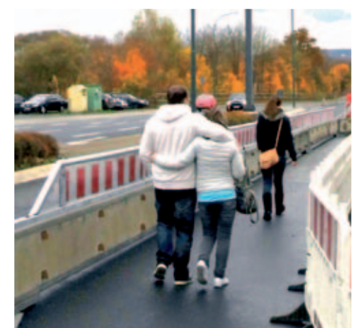
Safe footpath through the roadworks: mobile crash barrier ProTec 120 with splashguard and security obstacle.
