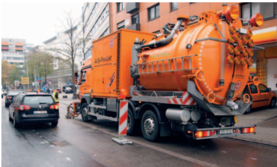
Without interrupting the flow of traffic, the AVS PeelJet removes hot- and cold-plastic road markings in Pforzheim town centre that are no longer needed after changing the road layout.
