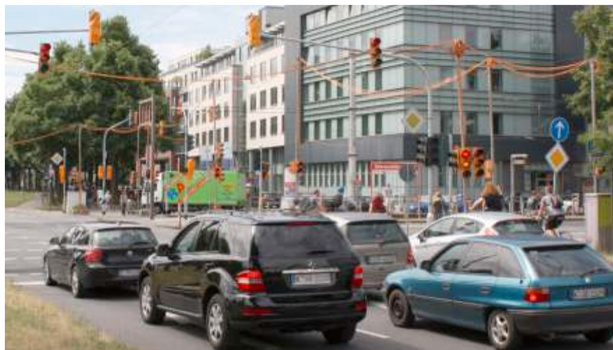
Major junction in Cologne: Innere Kanalstraße/Aachener Straße, traffic intersection with a mobile traffic light controller EPB 48 master and two remote slave controllers. Signal heads, buttons, radar detectors, camera systems, wiring, stands and overhead units - all by Berghaus, of course!
